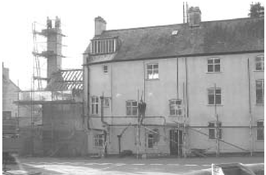
Demolition workers make a start on the chimney of the old laundry
